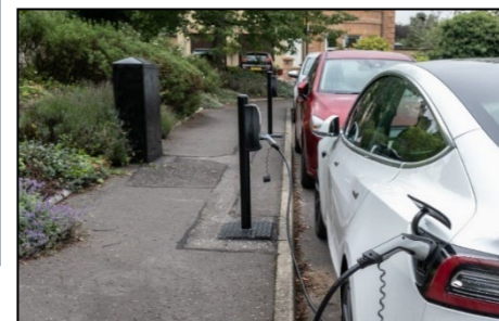
Figure 5.3 - 7-22kW On-Street Chargers
