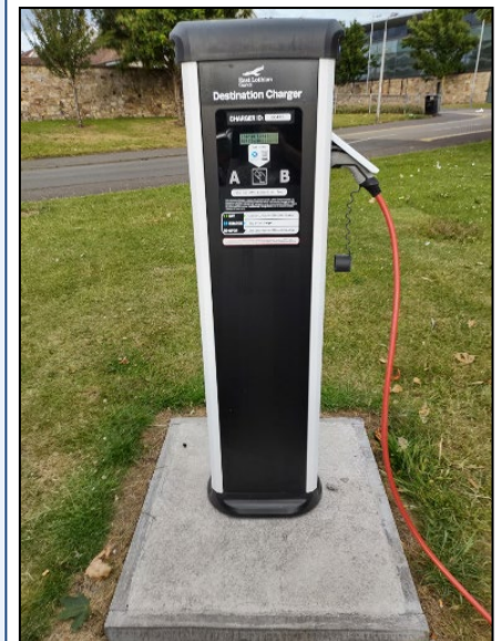
Figure 5.2 - 7-22kW Destination Charger
