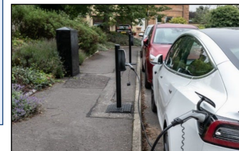
Figure 5.3 - 7-22kW On-Street Chargers
