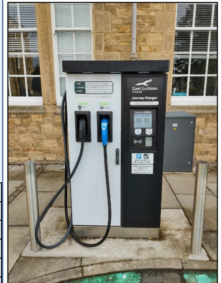
Figure 5.1 - 50kW Journey Charger
