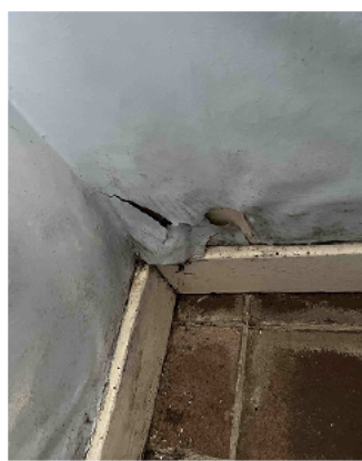
Fig. 3 Damp damage evident to internal walls
