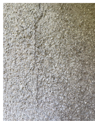
Fig. 4 Cracked render, possible lack of wall ties
