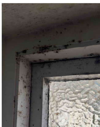
Fig. 2 Rotting window frames
