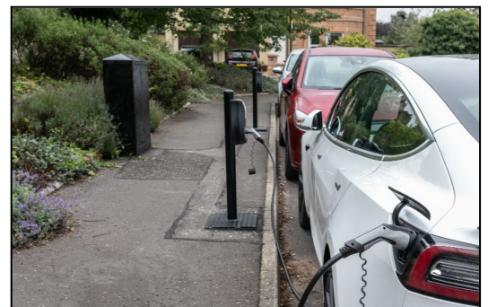
Figure 5.3 – 7-22kW On-Street Chargers
