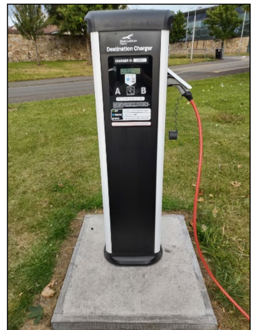
Figure 5.2 – 7-22kW Destination Charger
