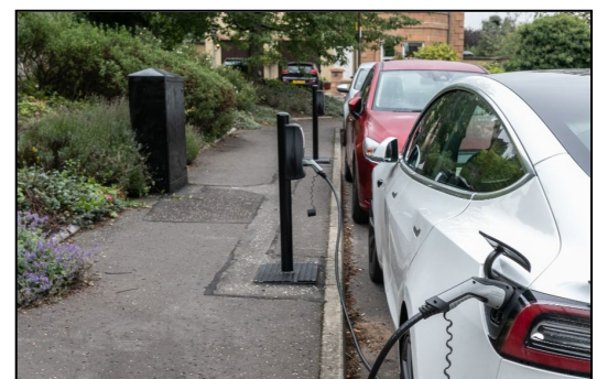
Figure 5.3 – 7-22kW On-Street Chargers
