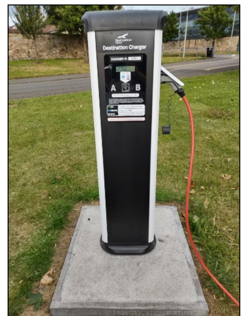
Figure 5.2 – 7-22kW Destination Charger
