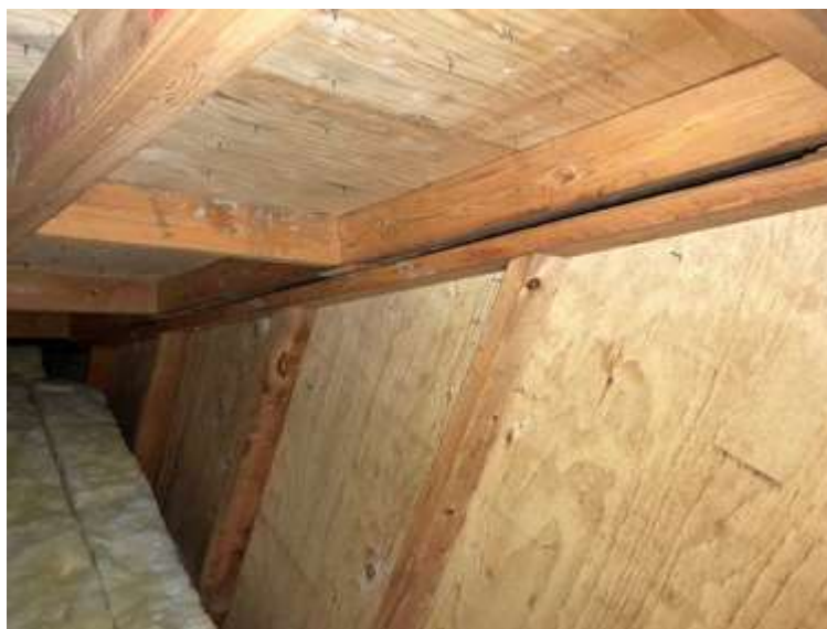
Gap and packers show poor tolerance between roof and wall head
