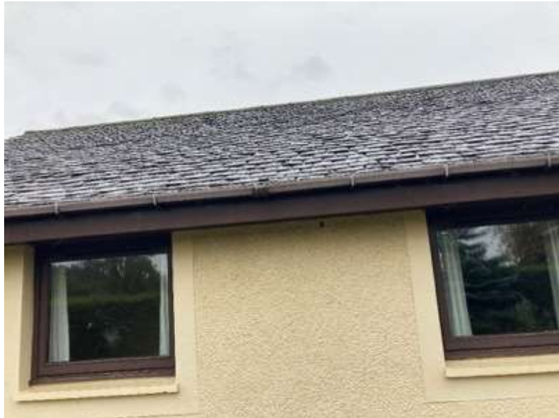
Uneven slate finish due to failing plywood sarking
