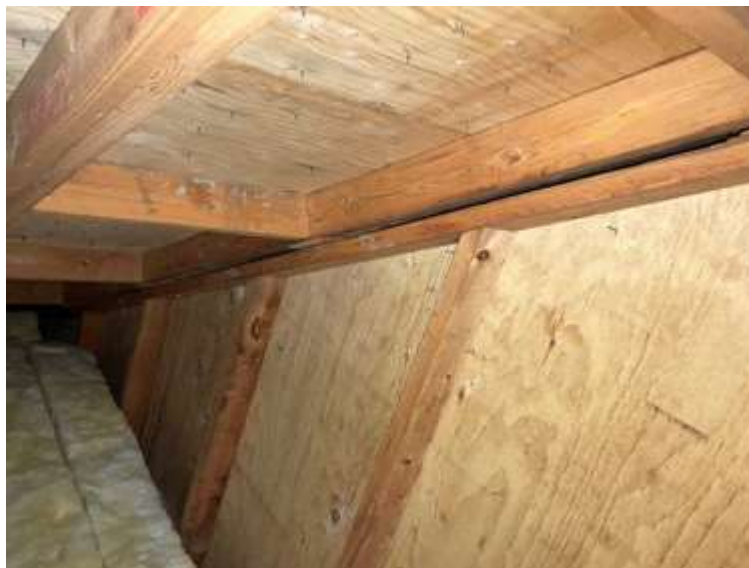
Gap and packers show poor tolerance between roof and wall head
