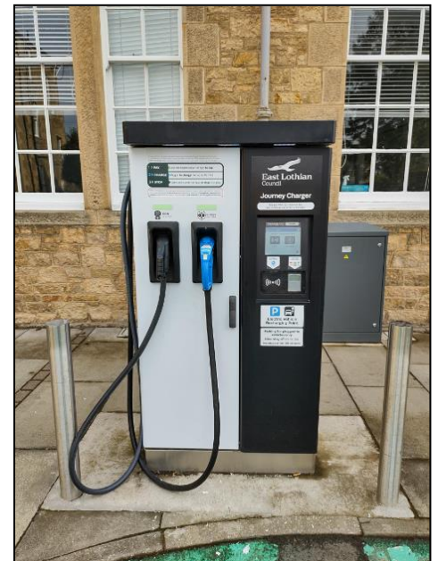
Figure 5.1 - 50kW Journey Charger
