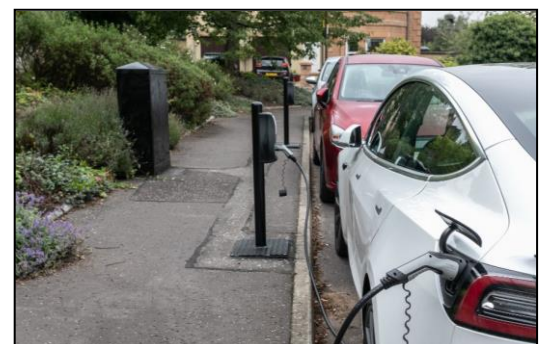
Figure 5.3 – 7-22kW On-Street Chargers
