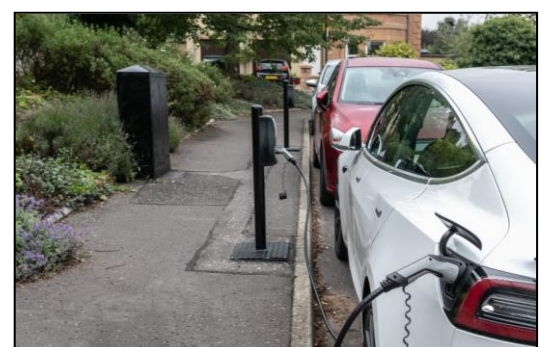
Figure 5.3 – 7-22kW On-Street Chargers
