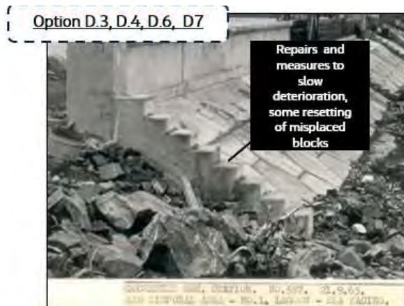
Figure 10 - (D.) Stepped Beam Short Listed Options D.3, D.4, D.6, D.7 indicative sketch
