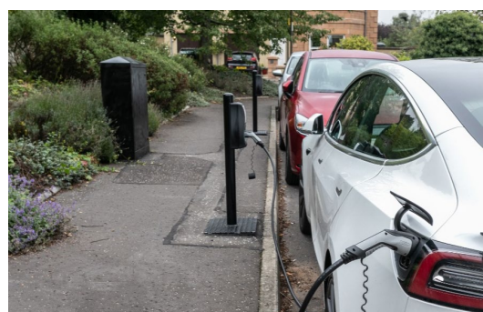
Figure 5.3 – 7-22kW On-Street Chargers
