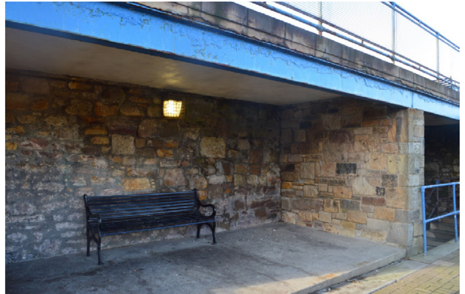
Existing viewing platform and shelter which is proposed to be removed as part of project brief
