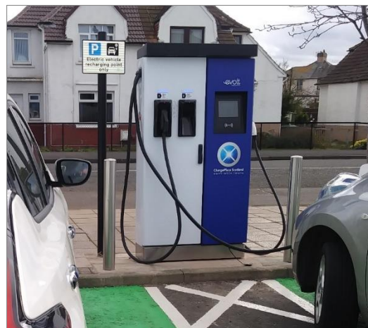
Figure 5.2 - Rapid 50kW DC Journey Charger
