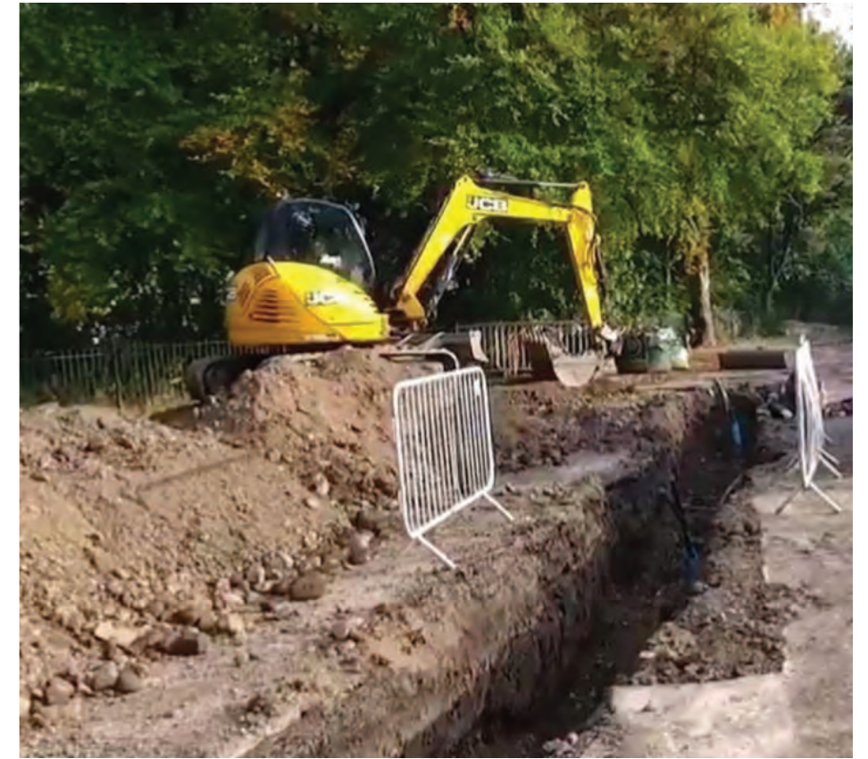
Installation of pipes for ground source heat pump at Saughton Park. Image credit: Pete McDougall / City of Edinburgh Council
