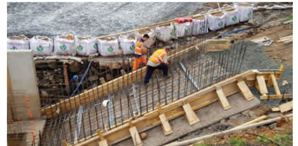
Installation of dam for micro-hydro at Saughton Park. Image credit: Pete McDougall / City of Edinburgh Council
