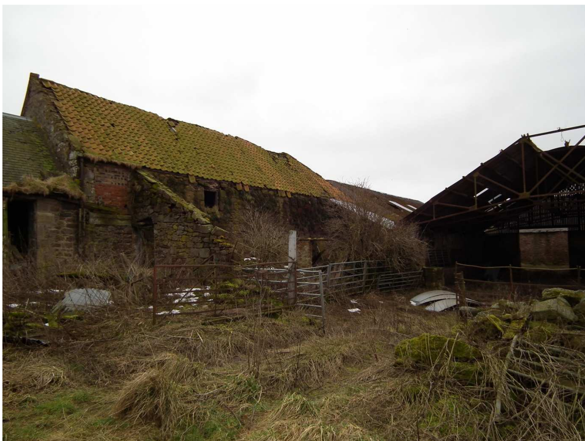
North Wall of Block D, Building G. East End of Building J.
