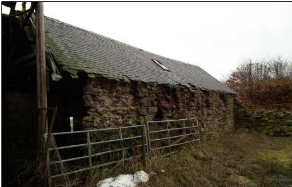
Fig 10: Building not structurally suitable for retention (location of detached new build)
