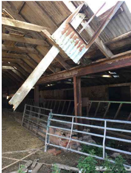
Collapsed roof, central portion
