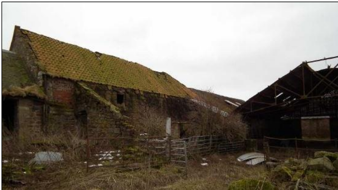
Fig 8: Building not structurally suitable for retention ('infill' new build, unit 8)
