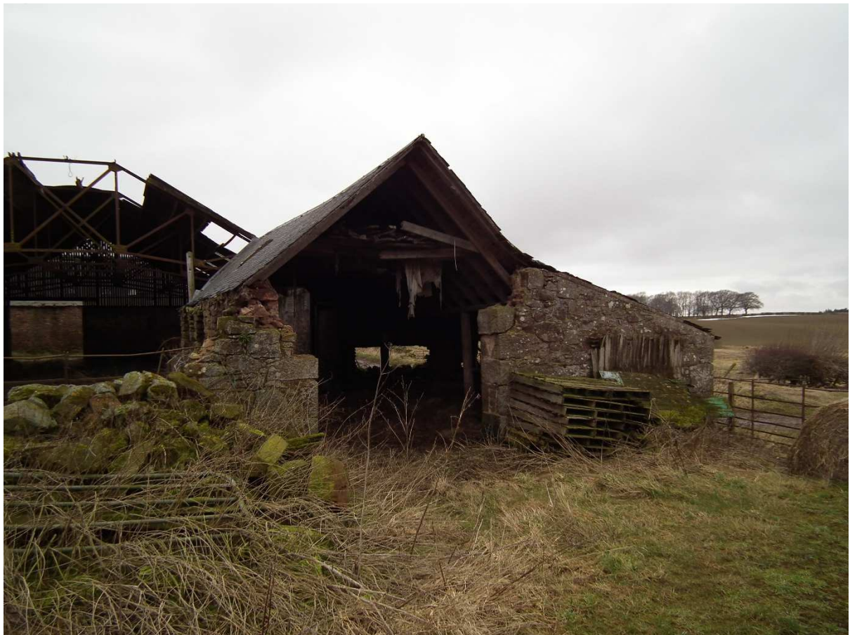
South Wall of Block E, Building H. East End of Building J.
