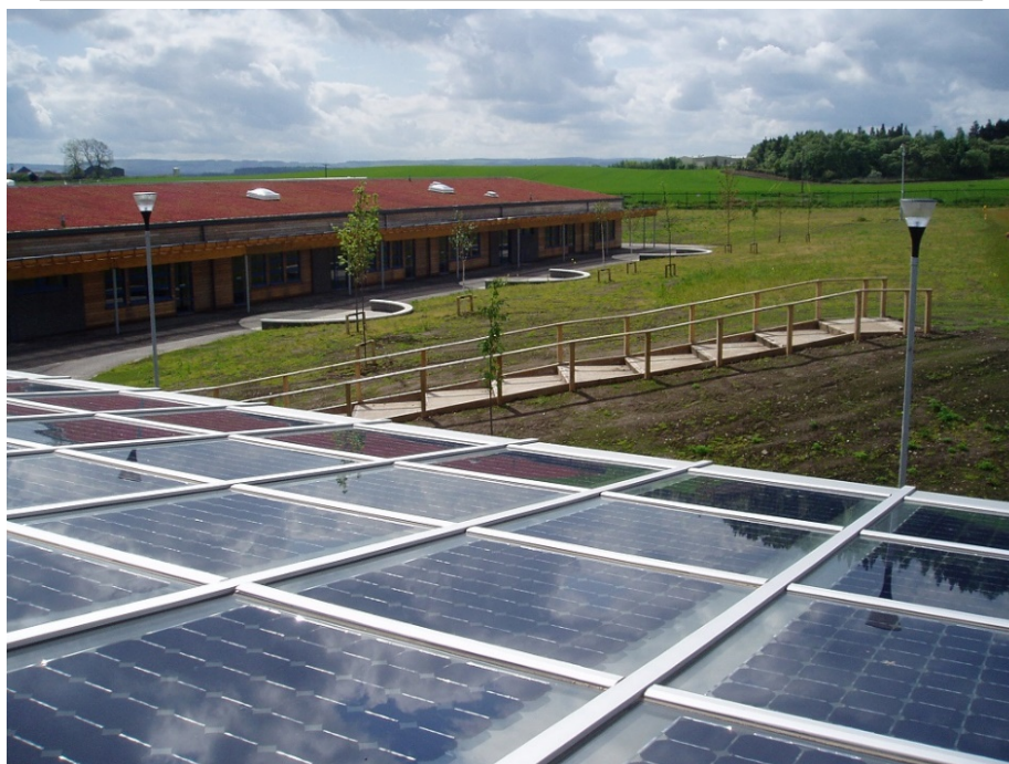
Figure 10: Solar panels on Windygoul Primary School, Tranent
