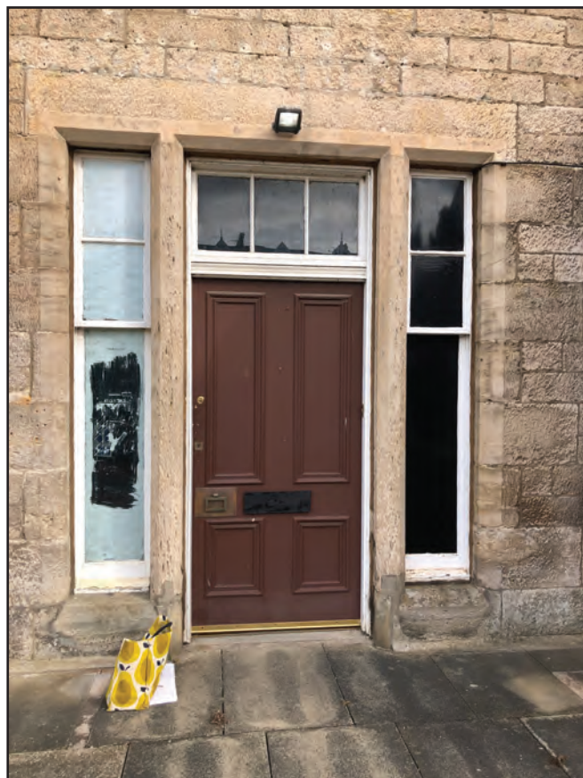
PLATE 2: No. 12 Westgate, detail of main entrance in the south elevation, from the south
