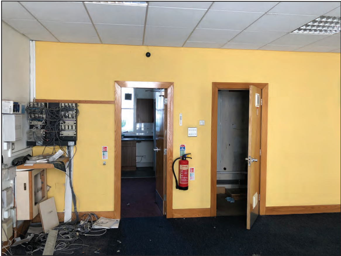
PLATE 9: Room 2, general view of the west side of the north wall, from the south
