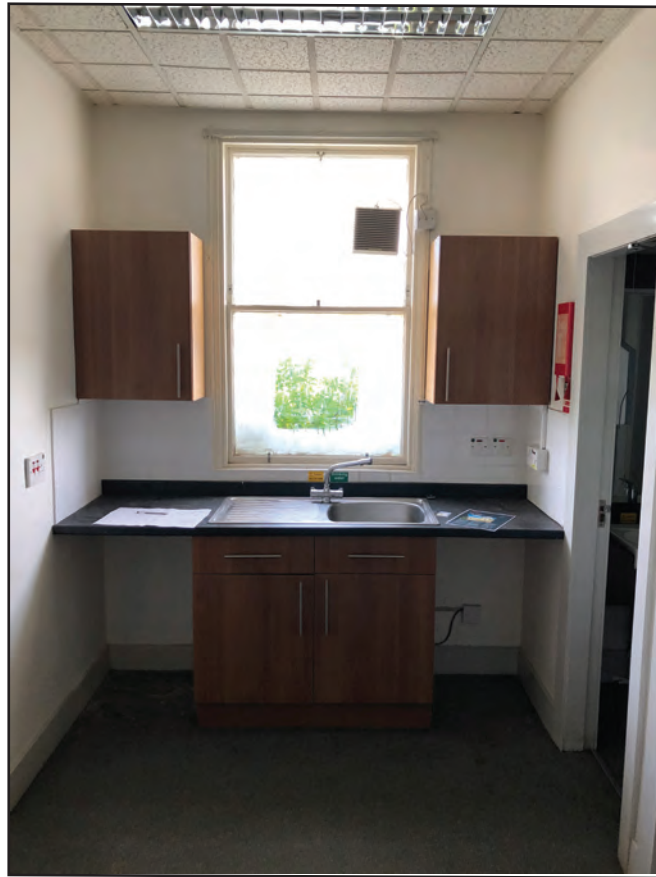
PLATE 11: Room 4, detail of the window in the north wall, from the south
