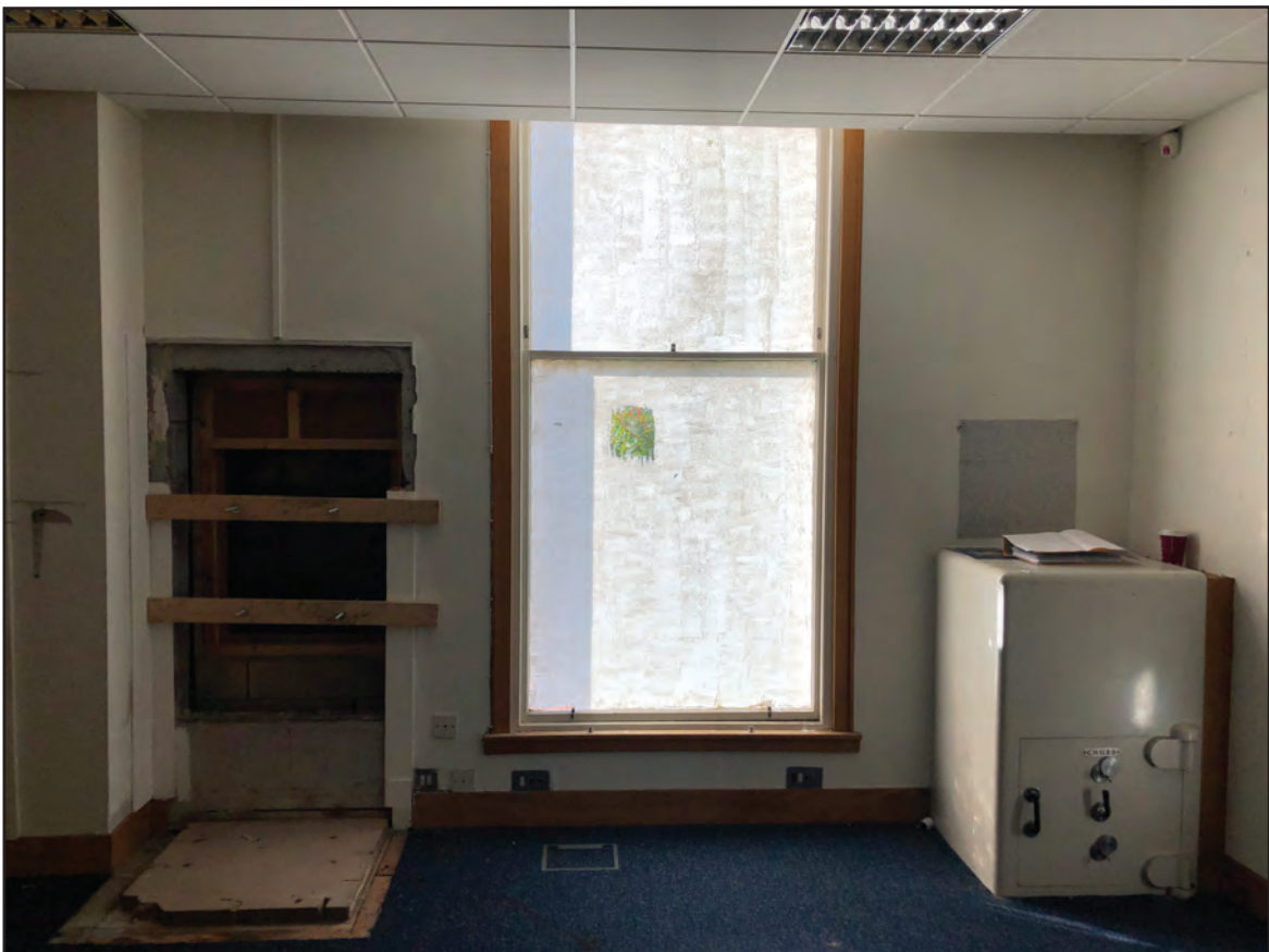
PLATE 10: Room 2, detail of the westernmost window in the south wall, disturbed by the false ceiling, from the north
