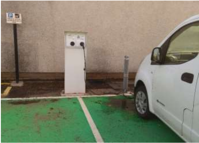
EVs charging points in Haddington. Credit: ELC
