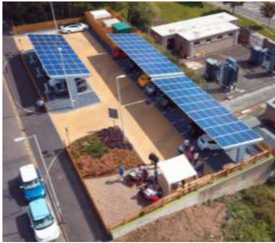
EVs charging hub Dundee. Credit: clean technica
