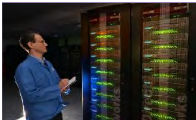
WCDI Computer Racks
