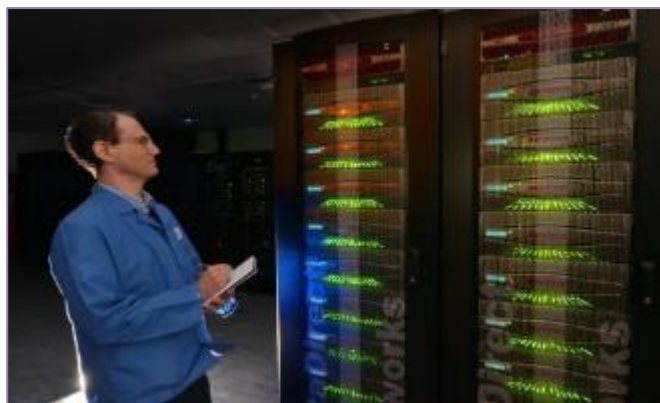
WCDI Computer Racks
