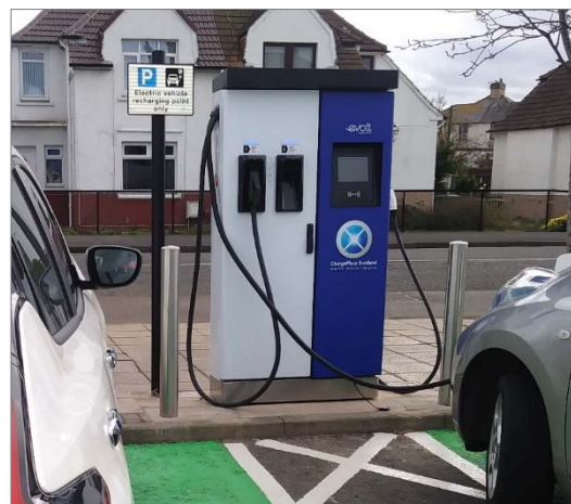
Figure 5.2 - Rapid 50kW DC Journey Charger
