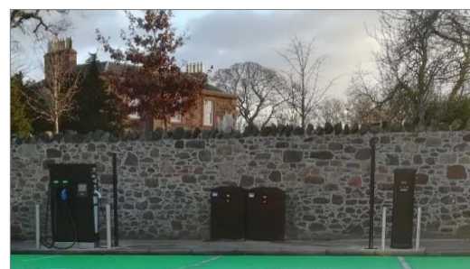
Figure 5.3 - Charging Hub in Conservation Area
