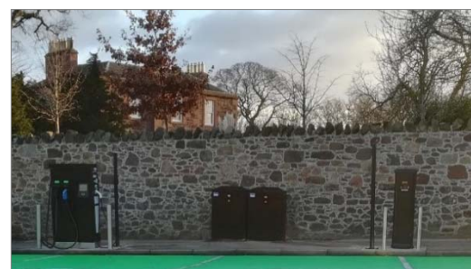
Figure 5.3 - Charging Hub in Conservation Area
