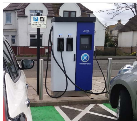
Figure 5.2 - Rapid 50kW DC Journey Charger
