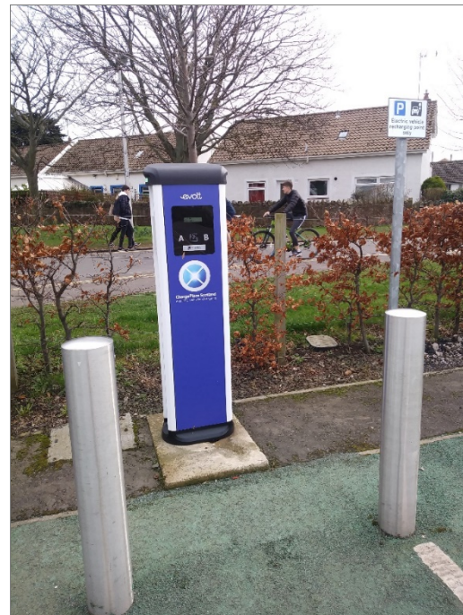
Figure 5.1 - 7-22kW AC Destination Charger
