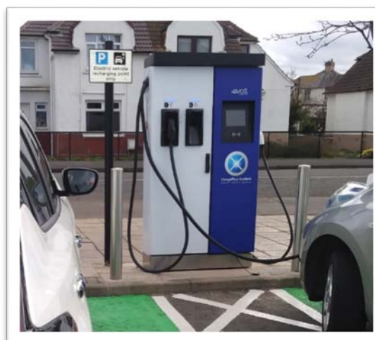
Rapid 50kW DC Journey Charger
