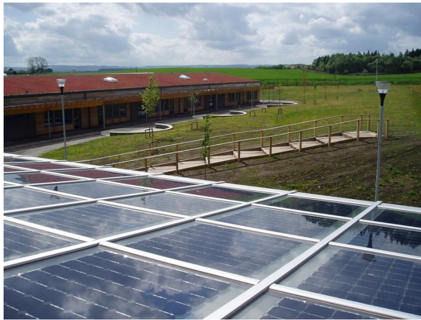
Figure 8: Solar panels on Windygoul Primary School, Tranent
