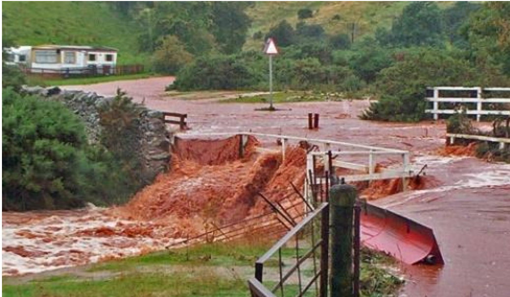
Figure 14: Flooded road in the Lammermuir Hills near Oldhamstocks
