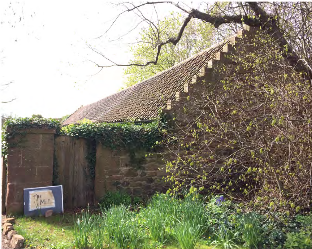
View of existing timber gate which is to be replaced from road A198. Gate attached to boundary wall which is listed.
