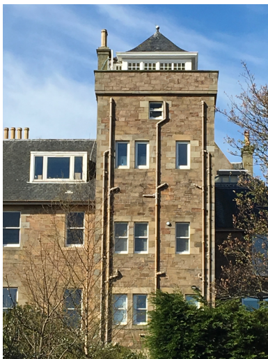
Photograph 4 The astragals to tower room windows are incongruous with the architectural style of the remaining property
