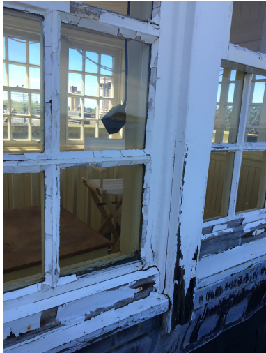
Photograph 3 Current condition of tower room windows due to weathering from exposed location
