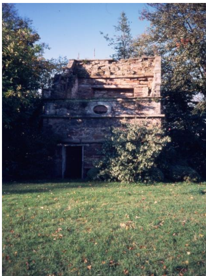
Figure 100 The listed doocot at Eskgrove requires repair
