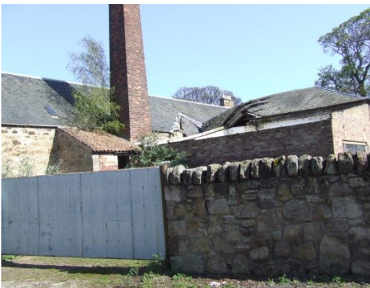
Figure 89 Pinkiehill Farm has deteriorated since becoming vacant
