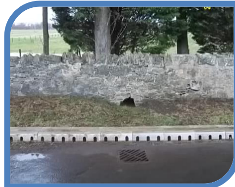
Road Drainage Infrastructure
