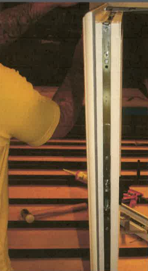
high security ironmongery used throughout
