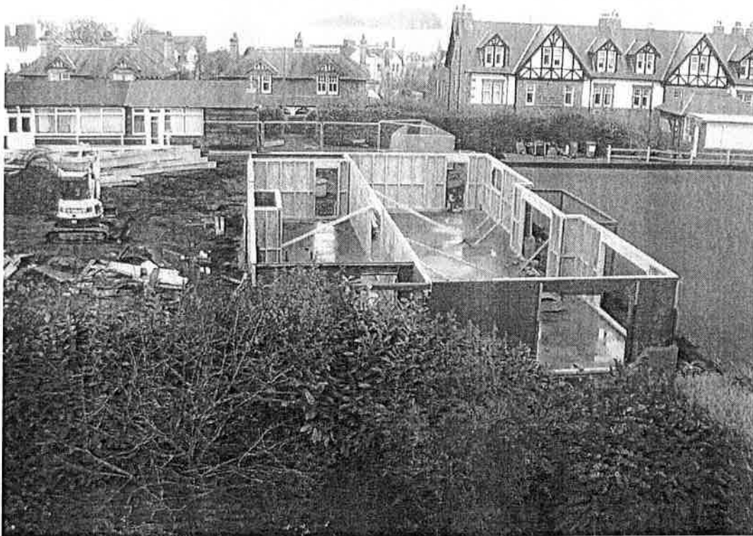
Photograph 1 :- View from Macnair Avenue showing the relative position of the old and new clubhouses. Planning consent allows for removal of the laurel boundary hedge.
