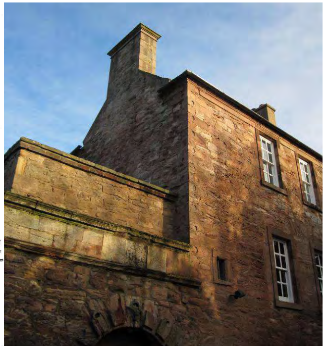
Fig. 16 House SW corner, showing buckled quoins, 2010
