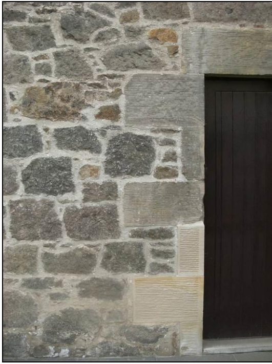
Photo ELC_12 P2: Detail of part of the north facing wall of the John Gray Centre, displaying irregular shaped porphyritic trachyte blocks making up most of the wall with shaped sandstone blocks forming the door surround. © BGS, NERC.
