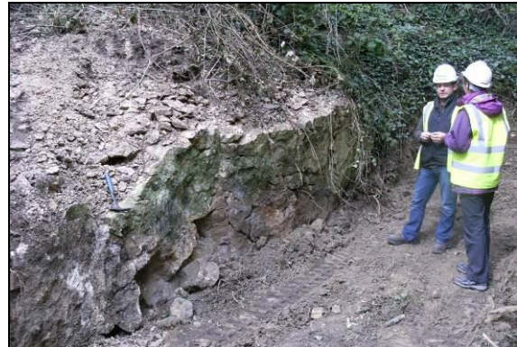
Photo ELC_12 P6: Ongoing work in the eastern part of the site has cleared material away the quarry face. Although the face will be left exposed, the floor is to be concreted and a fence constructed around the plot, impeding/preventing access to the exposure. Quarry face in the central part of the site. © BGS, NERC.
