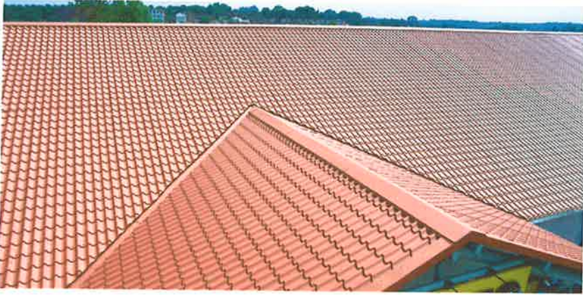
This is a profiled metal sheet roof on a supermarket in England
