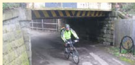
A bridge with sub-standard headroom on cycle route, Nottingham
