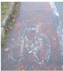
Facility ineffective due to poor maintenance
