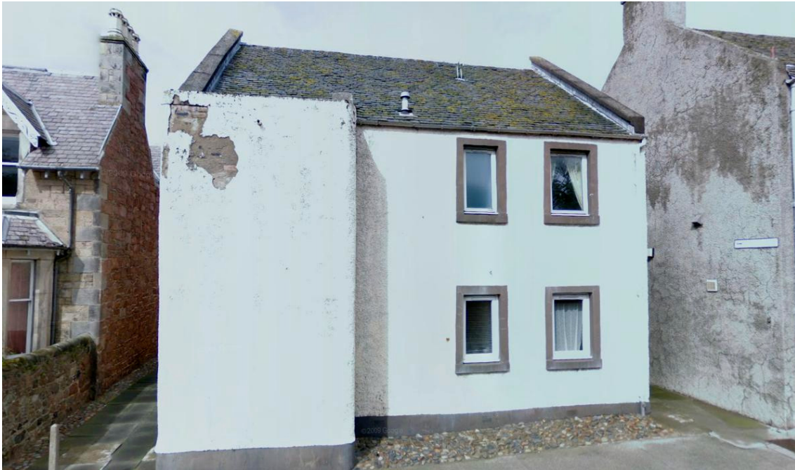
Above - PVCu windows in a property on East Road, off Balfour Street
