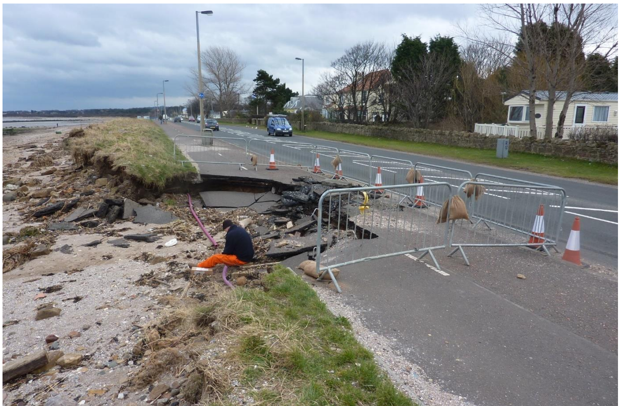
Coastal Erosion at Links Road Port Seton
